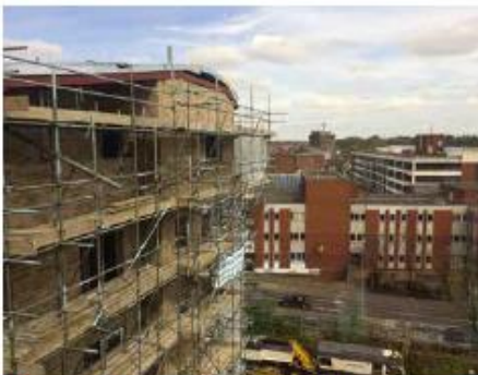
High density residential development at the former Pullman Tavern site in Grays
